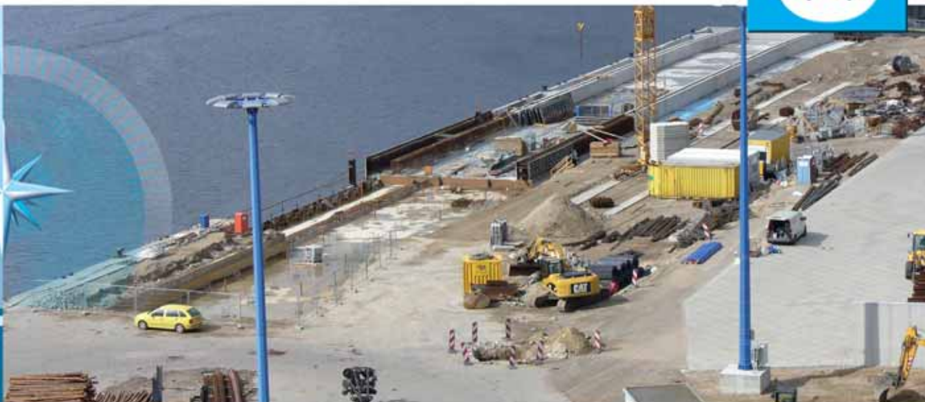
Building work at the port is in full swing, here in the area of berth 2.
